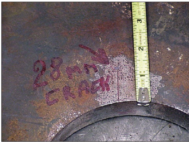
Figure 3-8: Cracked eye-bar of suspension bridge
