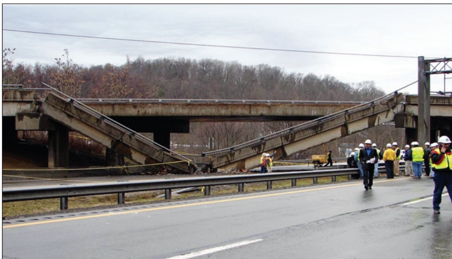
Figure 3-2: Box Beam Bridge Failure in Pennsylvania
