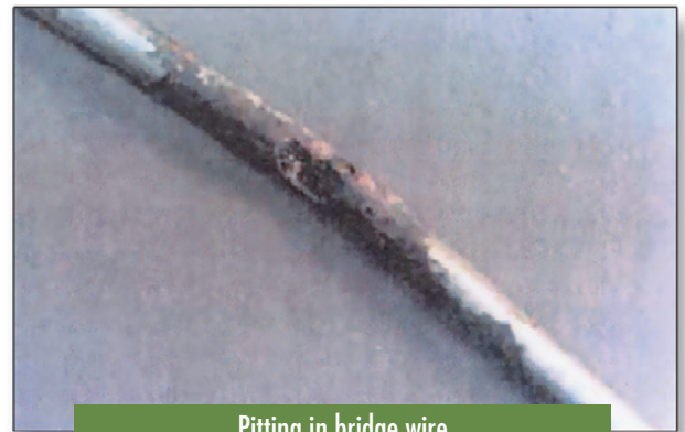
Pitting in bridge wire
