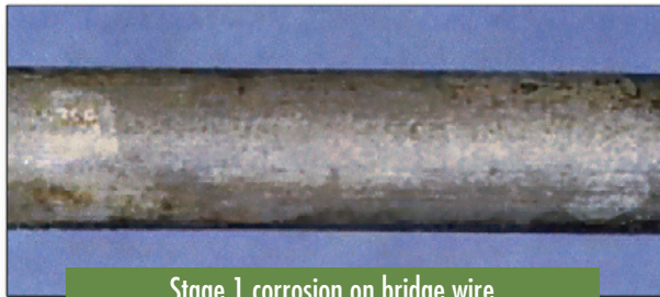
Stage 1 corrosion on bridge wire
