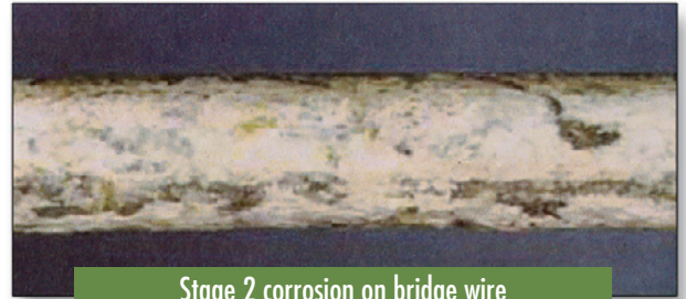
Stage 2 corrosion on bridge wire
