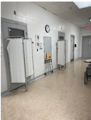
Exhibit 3. Two suicide observation rooms with detainees inside; the doors were covered with medical dividers, obscuring staff visibility of detainees in rooms, as OIDO observed on September 22, 2022.
