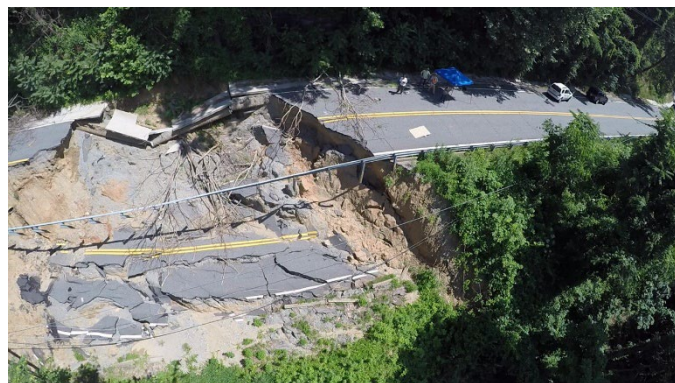
Landslide at Howard Gap Road, Hendersonville, NC. Photo: Jessica DeWitt, U.S. Geological Survey.
