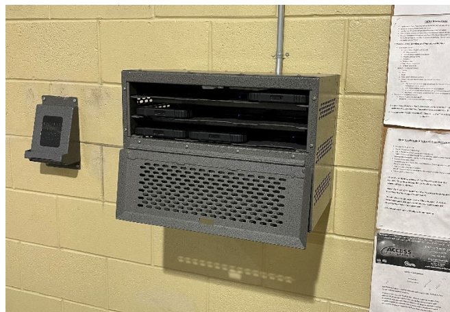
Exhibit 2. Talton wall unit and docking station, as OIDO observed on January 24-26, 2023.
