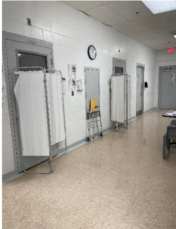
Exhibit 3. Two suicide observation rooms with detainees inside; the doors were covered with medical dividers, obscuring staff visibility of detainees in rooms, as OIDO observed on September 22, 2022.
