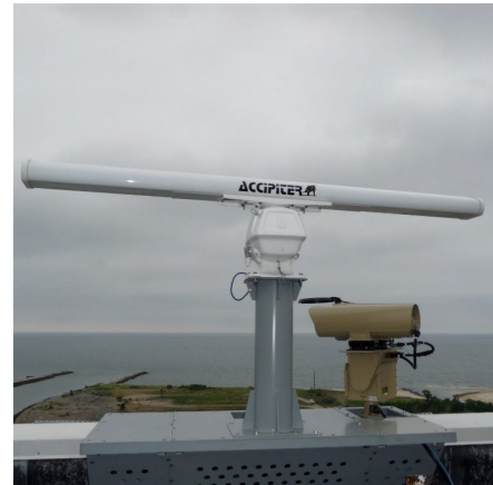
Figure 3-13 NM1-8A Security Radar
