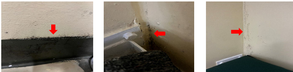
Exhibit 1. Black organic substance consistent with the appearance of mold on the lower wall in housing unit A-3 (left), black organic substance between corner walls of housing unit A-3 (middle), and black organic substance on the side wall of the housing unit A-3 (right), as observed by OIDO on June 27, 2023.
