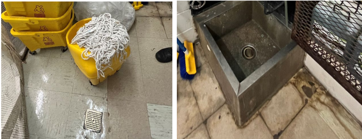
Exhibit 3. Drain on floor in chemical room showing that tile and drain are not flush with the rest of the floor (left); floor tiles in chemical room with broken and missing pieces (right), as observed by OIDO on September 26, 2023.
