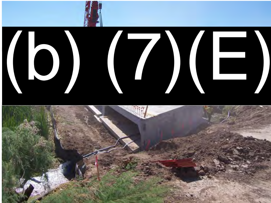
Whitewater Draw in Douglas Arizona Placement of the Precast Box Culvert by the National Guard Prior to Roadway Embankment Being Placed
