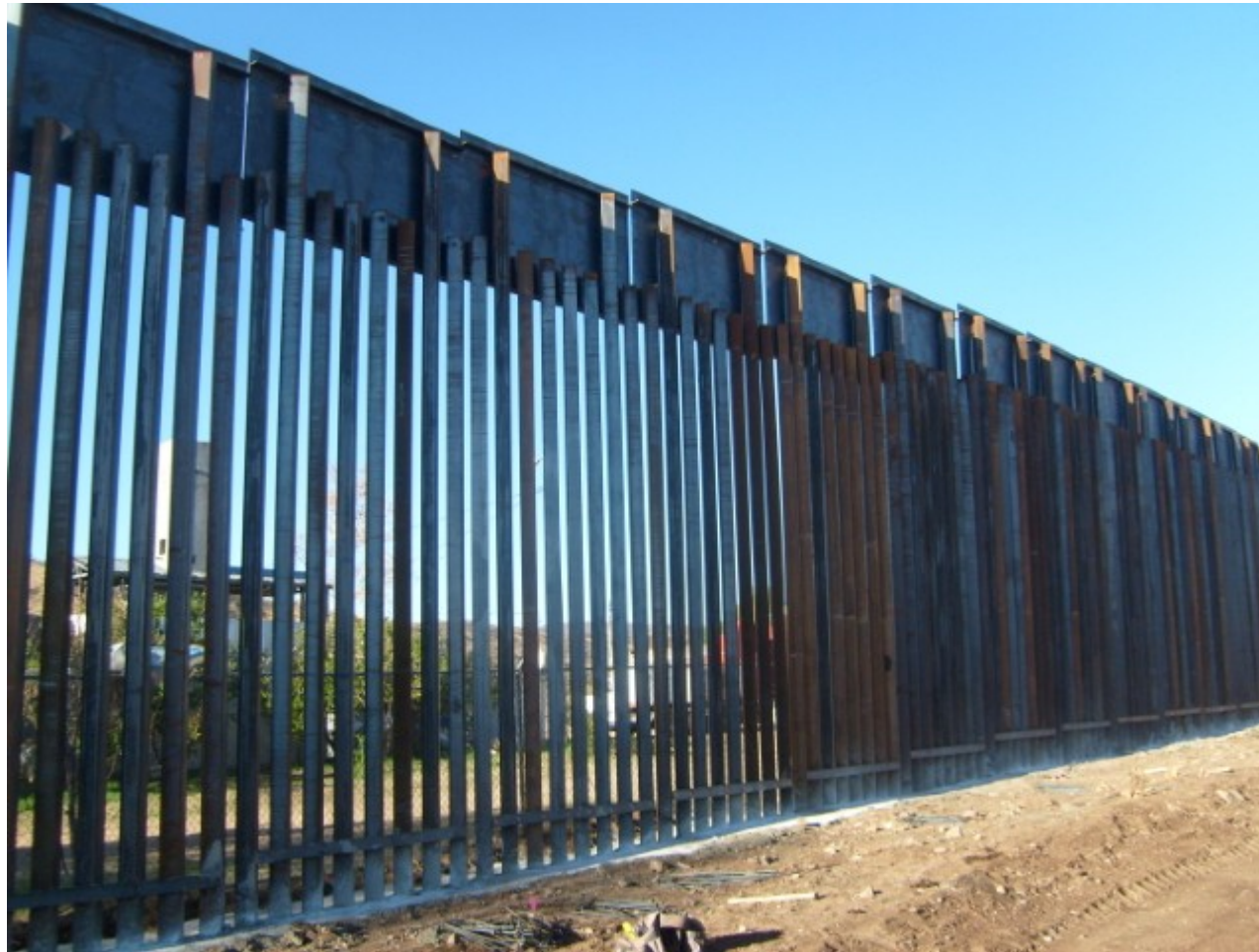
Pedestrian Fence – PV-1 Bollard Tucson Sector
