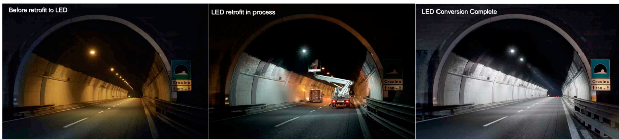
Figure 9: Before LED Retrofit
