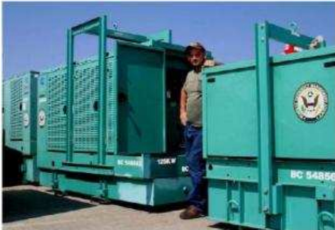
“Lifting Eyes” on the top and sides of these generators provide attachment points for crane rigging.
