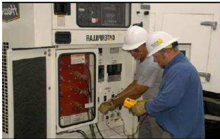
Operators check a 180 kW power generator used for powering an EOC.
