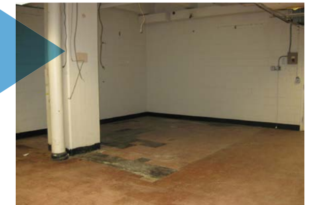
Static Electricity Shielded Room after.
