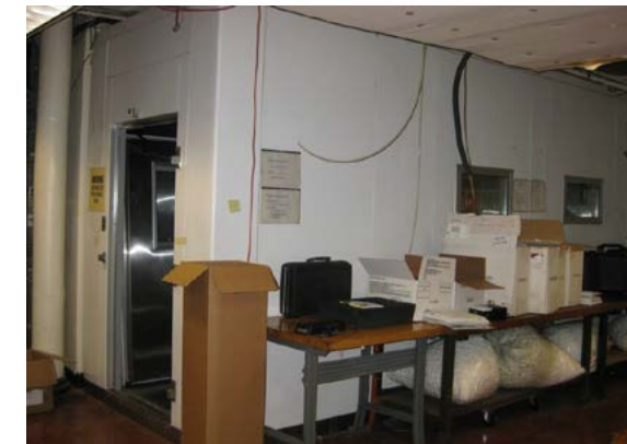
Static Electricity Shielded Room before.
