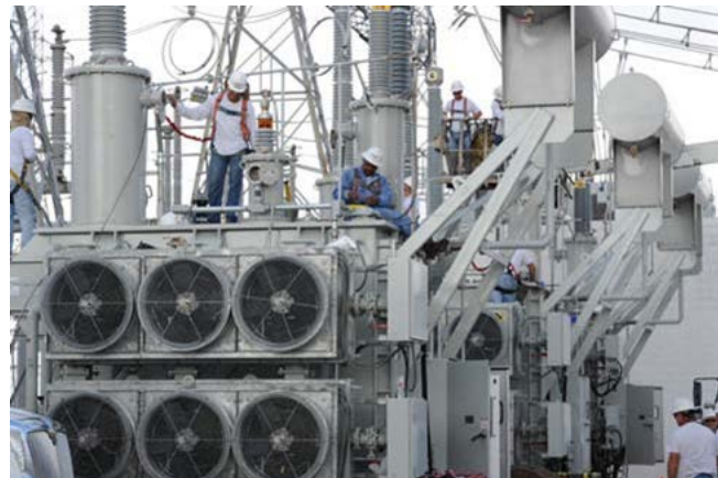
RecX in-grid deployment (Paul Wedig)
